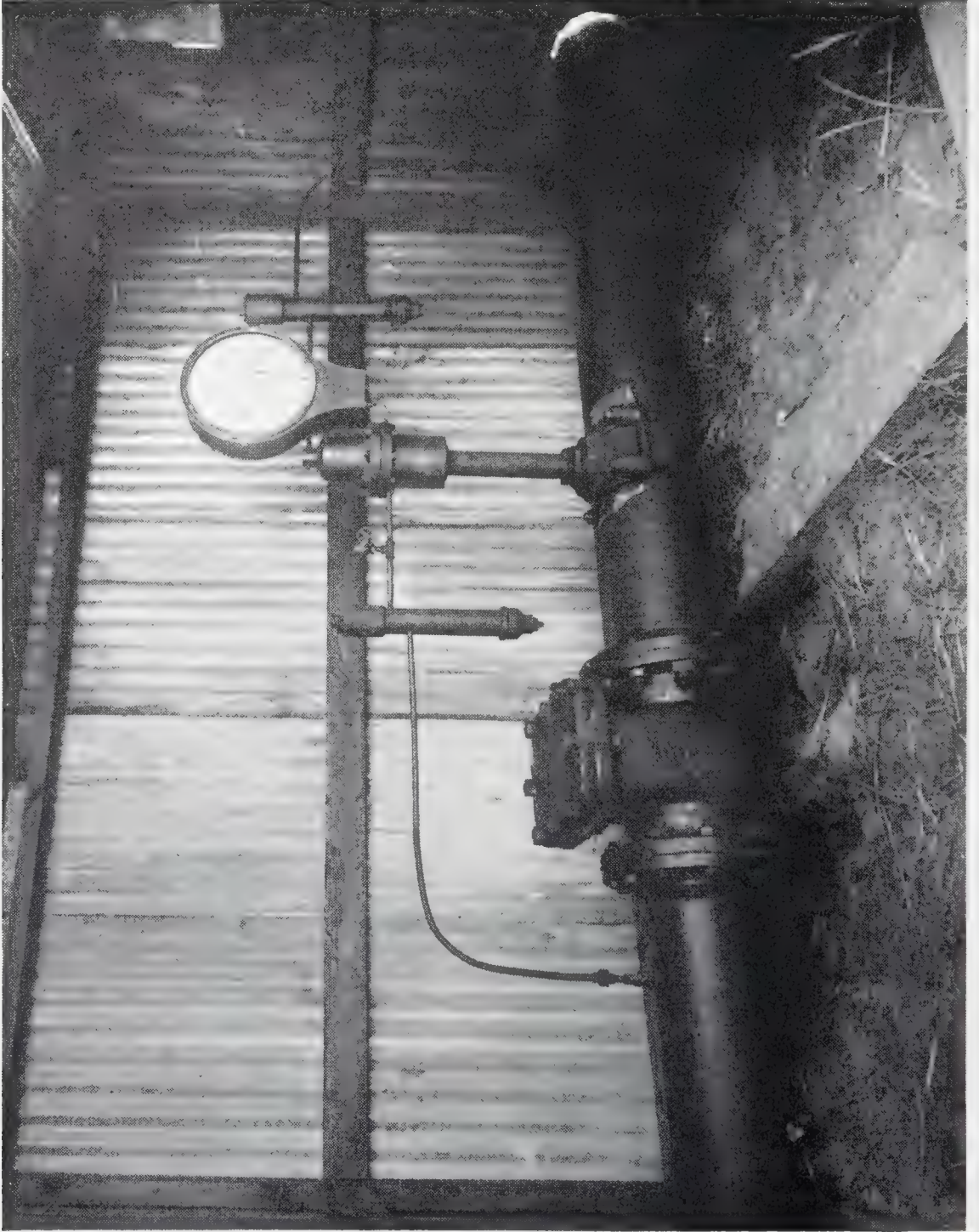
Fig. 95—ONE OF THE FIRST INSTALLATIONS OF ORIFICE METER BODY AND 50 INCH DIFFERENTIAL GAUGE
